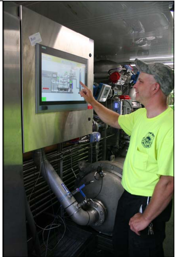
Park Ridge Water Department Operator Mark Gronbeck operating the controls on the new Purifics photo-catalytic advanced oxidation treatment system at Well 17.
