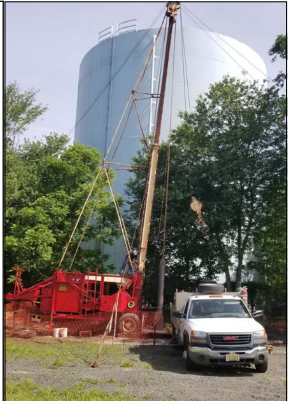
Contractor installing new 12" diameter groundwater well near the Holly Court Water Storage Tank. Well to be drilled to a depth of 350'. Pumping and Treatment facility planning and permitting has begun and is slated to be online in 2020.
